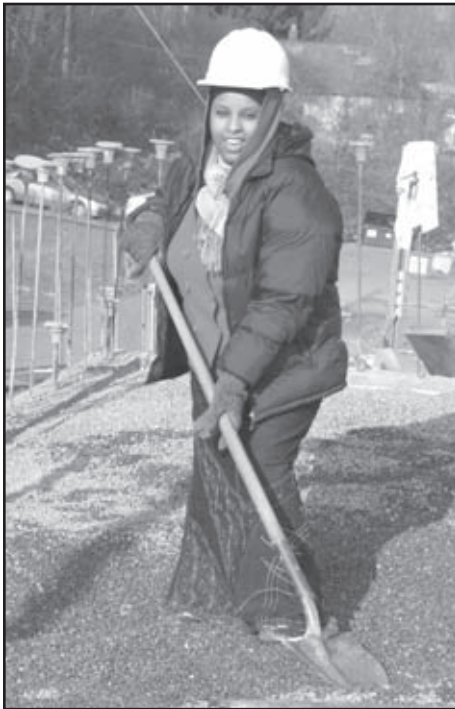
Khadra helps to fill in the foundation of her home in Rainier Vista.
